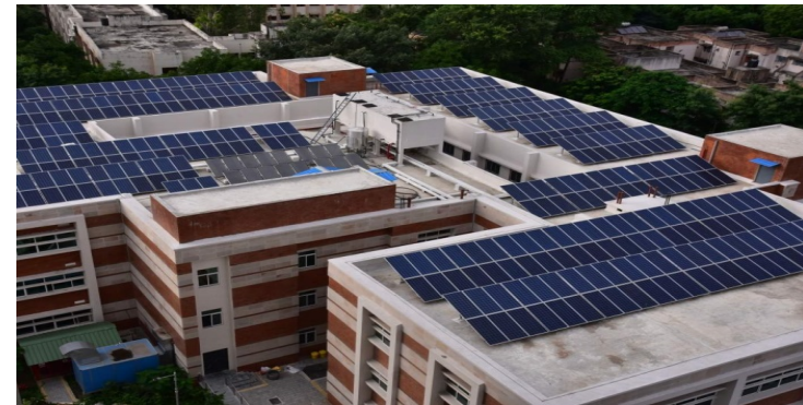
EPC for 4.8MW rooftop solar projects at Delhi, India
