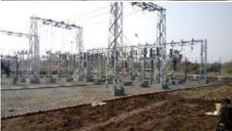
Electrical Infrastructure & Distribution Project
